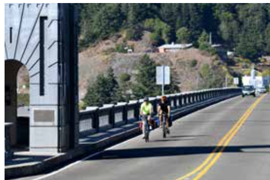
Narrow shoulders on the Isaac Lee Patterson Bridge over the Rogue River.
